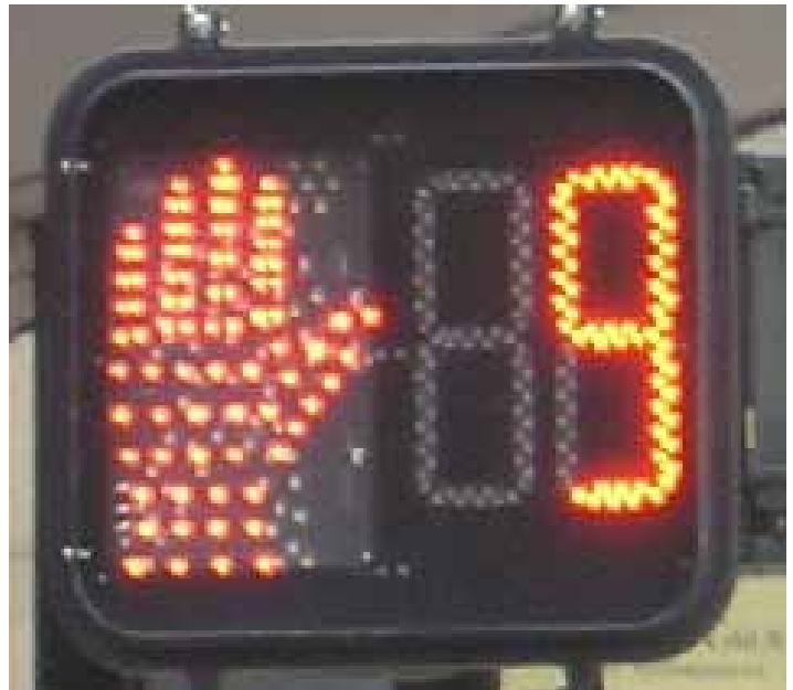
Pedestrian signals with countdown timers tell pedestrians how much time is left to cross the street.
